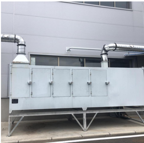
滤筒除尘器及活性炭净化箱
